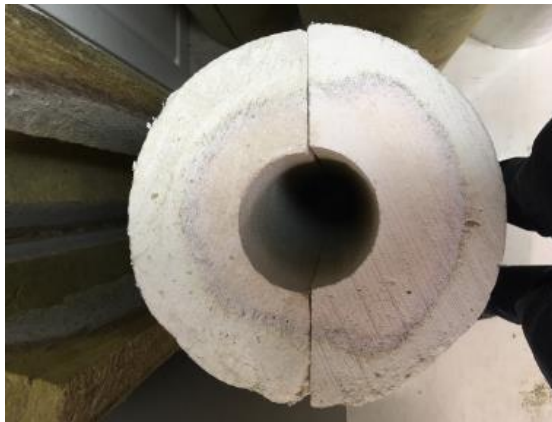
Calcium silicate after high temp exposure
